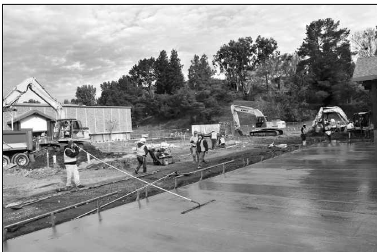
Work is in the final stages on the new central courtyard at Rossmoor Shopping Center.
